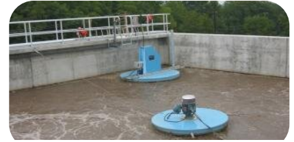
Aeration & Mixing / SBR
