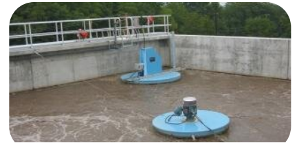
Aeration & Mixing / SBR
