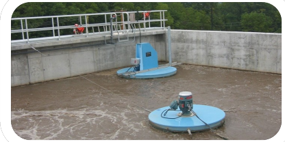
Aeration & Mixing / SBR
